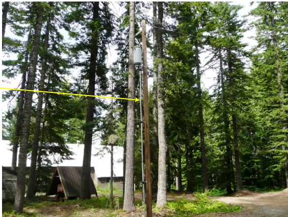
New pole at the maintenance shed (also known as the Zoo)
