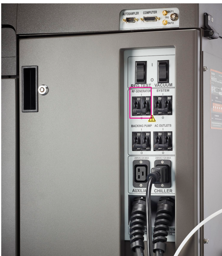
Figure 30. The RF generator circuit breaker on the Helios circuit breaker panel
