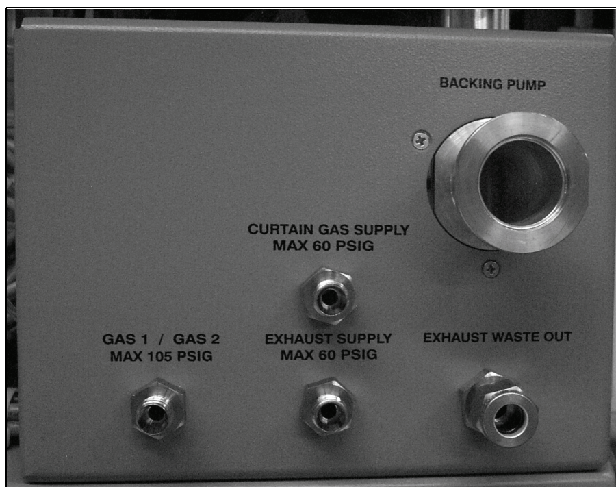
Gas and vacuum panel
