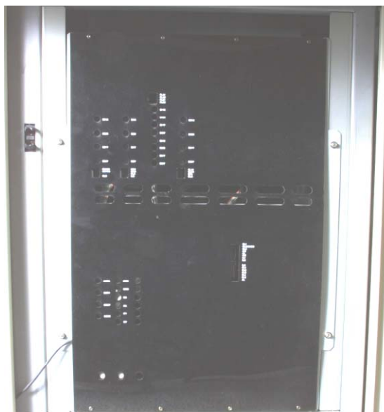
Fig. 4.6 Control panel R2
