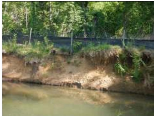
Highly eroded bank along Tuscarora Creek.
