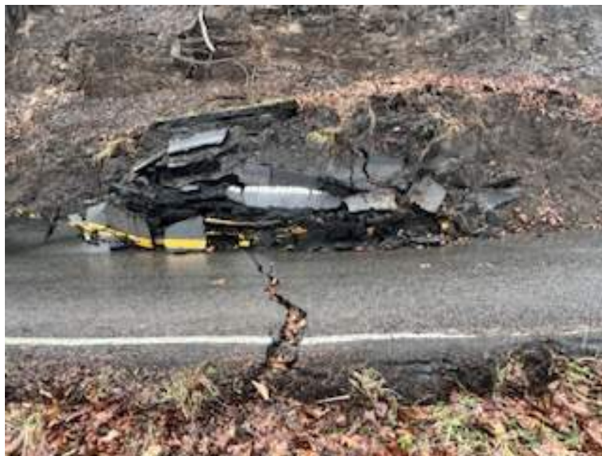
Figure 647: Damage from Landslide Event on Route 91
