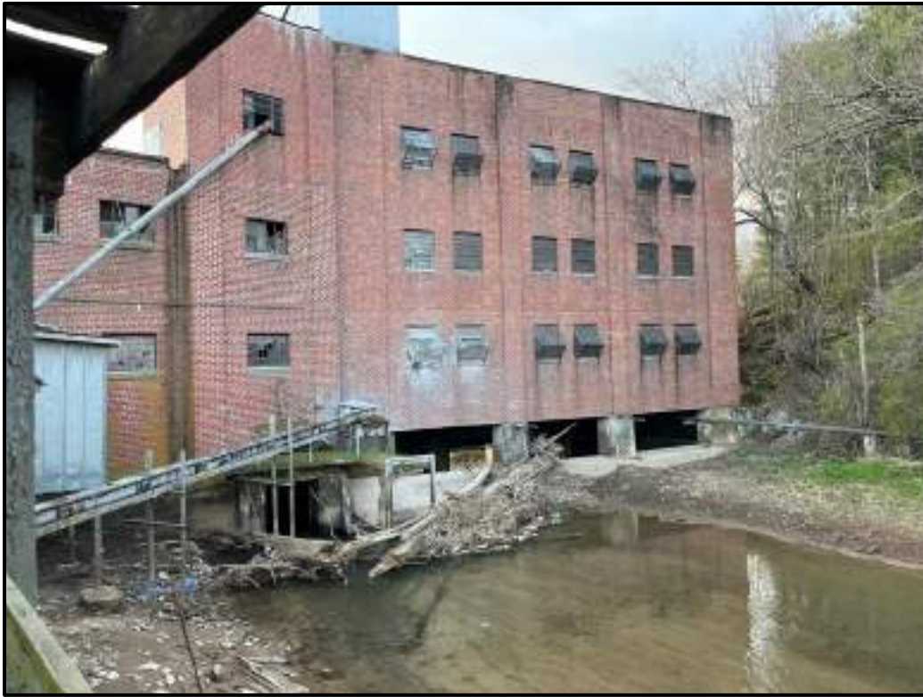
Figure 71: Mill Building March 2023 capturing debris
