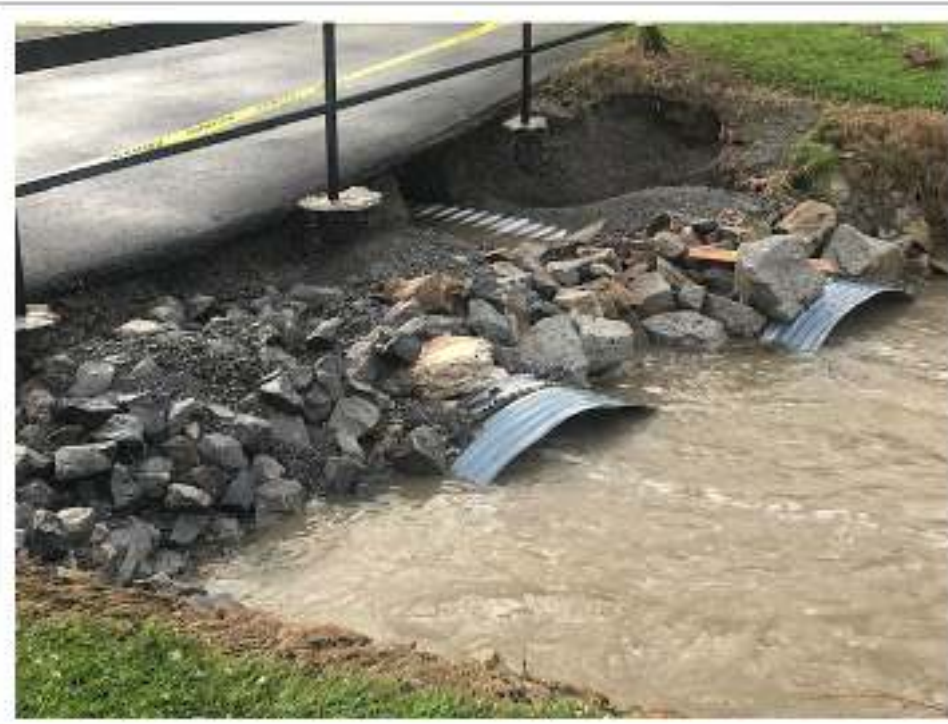
Photo 1: L.F. Addington School Bus Bridge Damage (2019)
