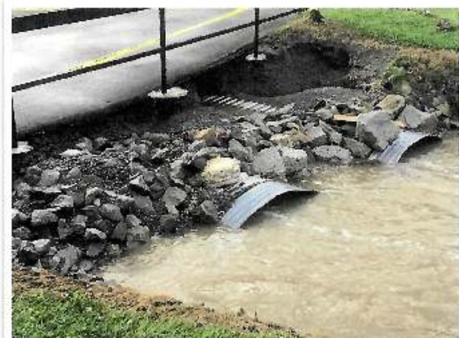
Photo 1: L.F. Addington School Bus Bridge Damage (2013)
