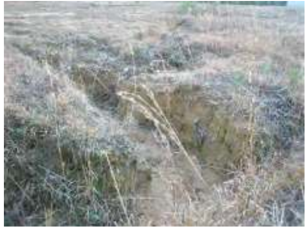
Figure 2: Erosion of outlet
