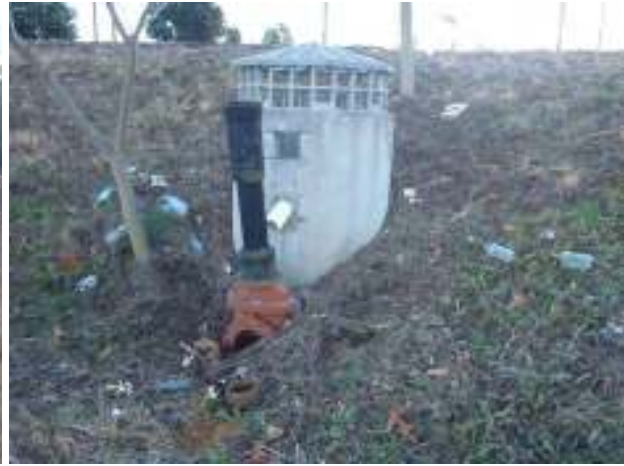
Figure 2: Trash around outlet structure
