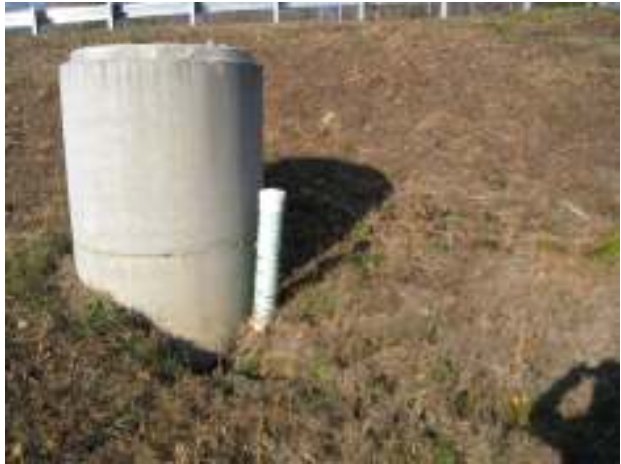
Figure 4. Basin outlet, with erosion at base
