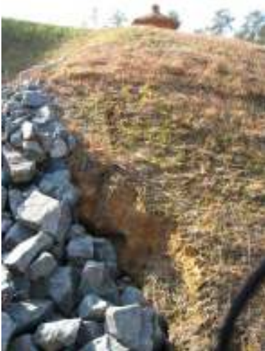
Figure 5. Steep basin inlet, eroding
