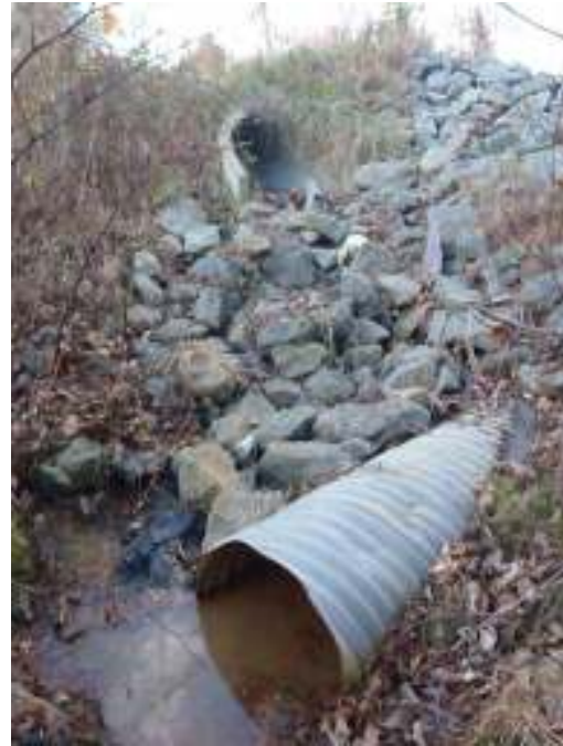
Figure 2: Metal outlet pipe partially clogged
