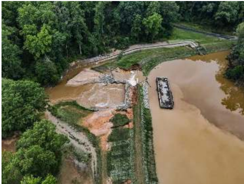
Figure 6-18: Dam Failure at Chandlers Mill Dam
