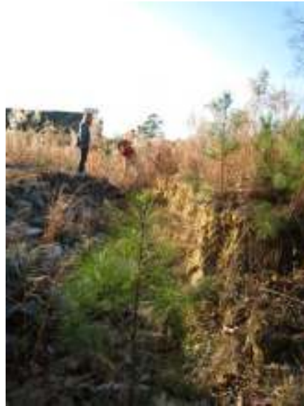
Figure 2: Dam section eroded out at spillway
