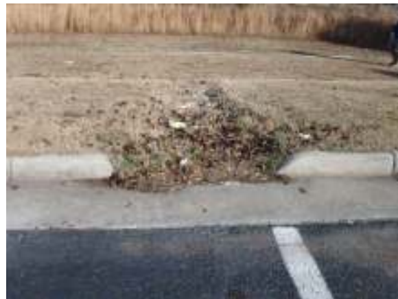
Figure 3: Partially clogged inlet to basin
