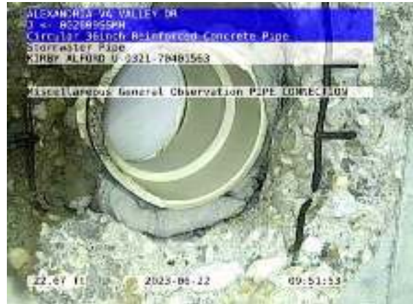
009388STMP_b794ec58-abe6-4011-9022-35b8449e26a7_20230622_102442_561.jpg, 00:00:56, 22.68ft Miscellaneous General Observation / PIPE CONNECTION
