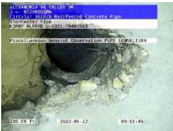
009388STMP_0ab3cd11-735a-406a-935f-63c88756cb4f_20230622_102834_872.jpg, 00:04:20, 210.65ft Miscellaneous General Observation / PIPE CONNECTION
