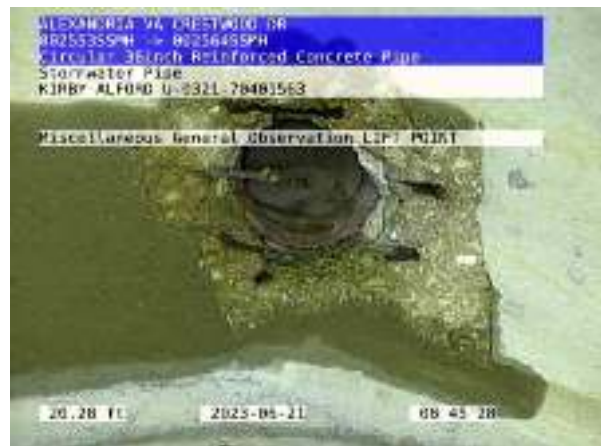
007464STMP_4e6de127-f280-4387-bf53-1f96ddb88169_2023 0621_091815_311.jpg, 00:01:08, 20.28ft Miscellaneous General Observation / LIFT POINT
