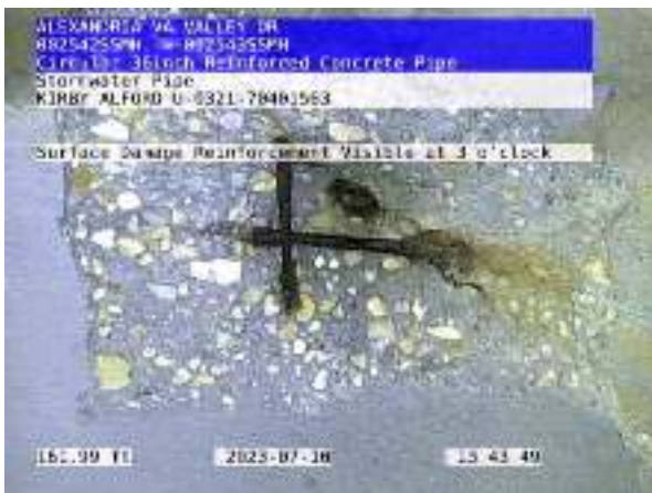
009180STMP_6f5bfa64-b2f4-4464-a473-43d7d9ee9cb2_2023 0710_141717_416.jpg, 00:03:38, 161.99ft Surface Damage Reinforcement Visible at 3 o'clock
