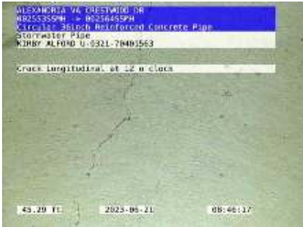
007464STMP_bb3d9554-8eb0-4290-a689-0782eaa1fdcf_20230621_091904_422.jpg, 00:01:51, 45.29ft Crack Longitudinal at 12 o'clock
