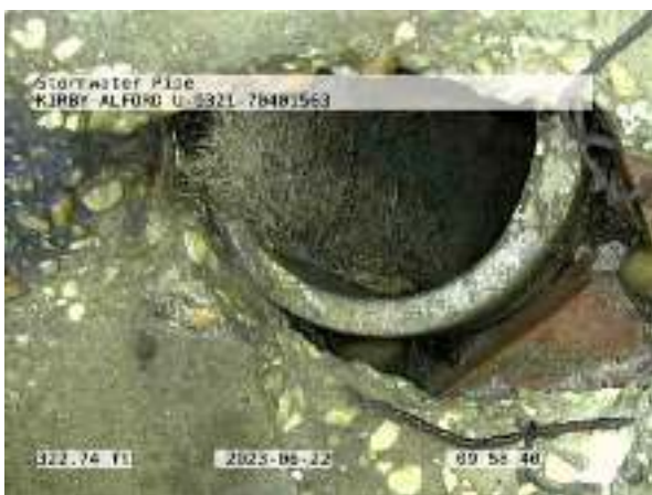
009388STMP_5ebd683e-711c-49d0-a262-69ebe03f0d01_20230622_103130_145.jpg, 00:06:51, 322.74ft Miscellaneous General Observation / PIPE CONNECTION
