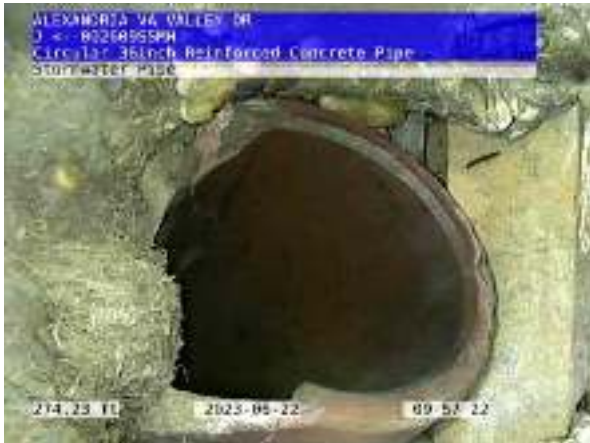
009388STMP_0977b09a-5761-4be2-a487-c69218e67a77_20230622_103012_136.jpg, 00:05:45, 274.23ft Miscellaneous General Observation / PIPE CONNECTION
