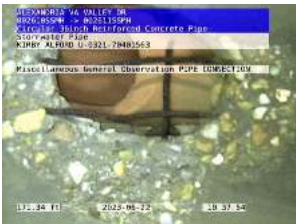
008792STMP_56783154-0477-4d56-81a9-b8e961aefbbc_20230622_111044_358.jpg, 00:03:51, 171.34ft Miscellaneous General Observation / PIPE CONNECTION
