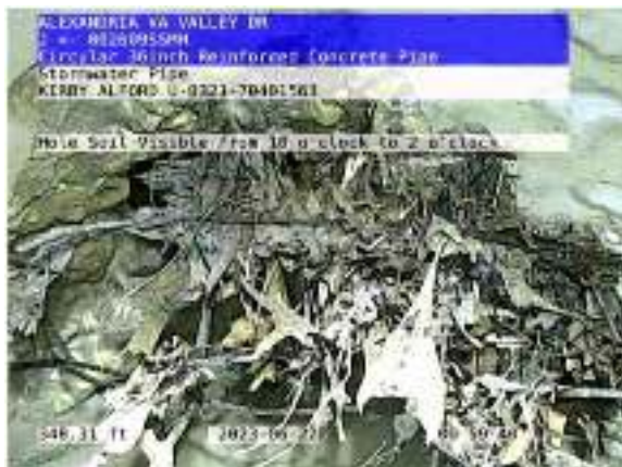
Photo 6: Hole visible in pipe 009388STMP
