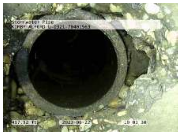
009388STMP_86105d55-416f-462b-9d92-d490a1984c71_20230622_103419_574.jpg, 00:09:04, 417.92ft Miscellaneous General Observation / PIPE CONNECTION
