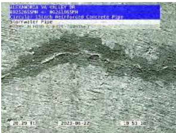
009391STMP_1e1a5cb9-f3d9-45f1-bdd9-9c8380fa6f5c_20230622_112407_985.jpg, 00:00:48, 20.29ft Crack Circumferential from 12 o'clock to 12 o'clock
