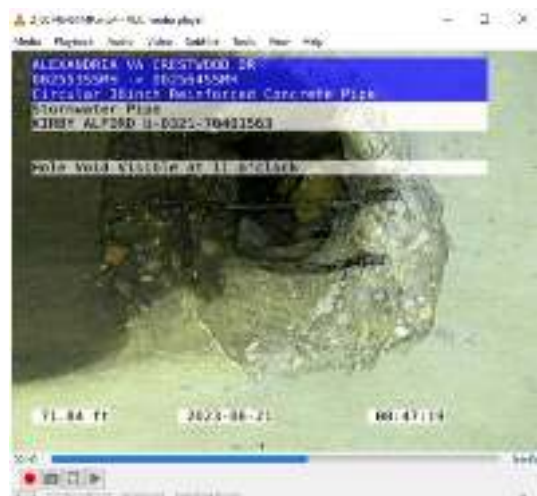
Photo 7: Broken pipe section in 07464STMP
