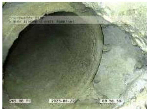
009388STMP_ca042ab8-bd12-4237-a815-a79c8a08b941_20230622_102947_852.jpg, 00:05:28, 265.86ft Miscellaneous General Observation / PIPE CONNECTION
