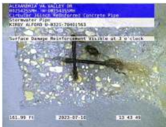
Photo 9: Surface damage visible in pipe 009180STMP
