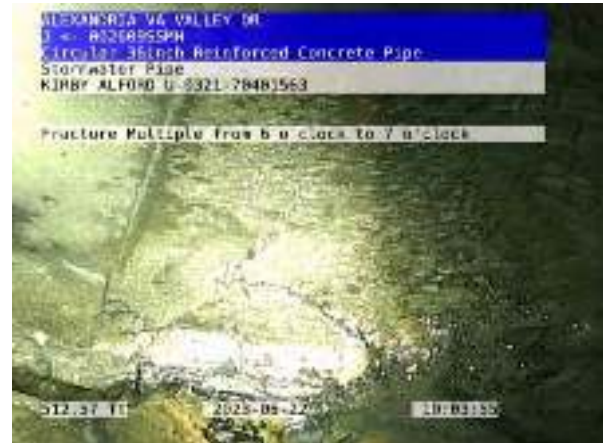
009388STMP_1c332d5d-e69f-40f5-bf2e-952484668de6_20230622_103644_924.jpg, 00:11:14, 512.56ft Fracture Multiple from 6 o'clock to 7 o'clock
