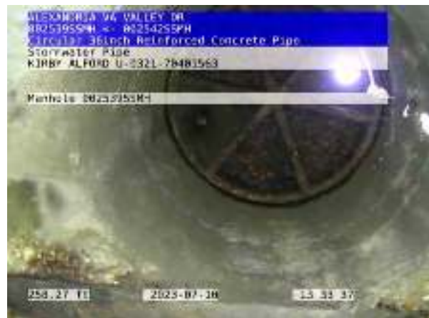
009066STMP_3b0af0b3-f9b7-4276-b462-81b09c5d994c_20230710_140706_010.jpg, 00:05:08, 258.27ft Manhole / 002539SSMH
