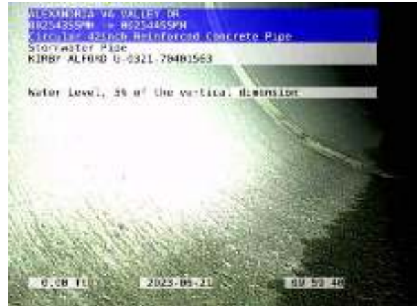
009181STMP_66f65b7b-6bf8-4116-bd99-0724494522f1_2023 0621_103227_957.jpg, 00:00:14, 0.00ft Water Level, 5% of the vertical dimension
