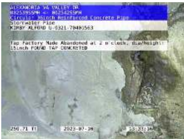
009066STMP_12888b6e-1916-4f20-a171-5b480e25d747_20230710_140644_835.jpg, 00:04:49, 250.71ft Tap Factory Made Abandoned at 2 o'clock, dia/height: 15inch / FOUND TAP CONCRETED
