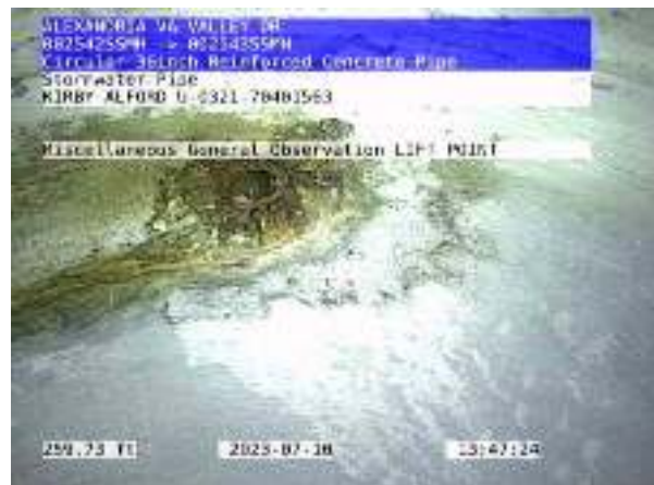
009180STMP_ed38141f-6705-44c0-b090-403b08637c30_2023 0710_142052_313.jpg, 00:06:47, 259.73ft Miscellaneous General Observation / LIFT POINT
