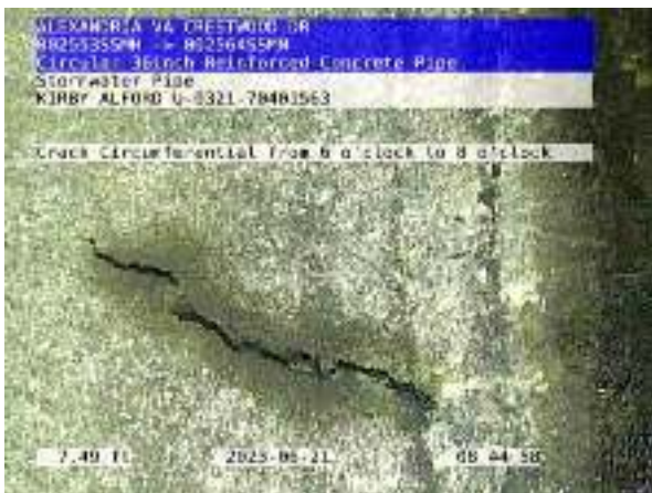
007464STMP_aa3425a4-f565-40ad-b4a5-371804118181_202 30621_091745_961.jpg, 00:00:44, 7.49ft Crack Circumferential from 6 o'clock to 8 o'clock
