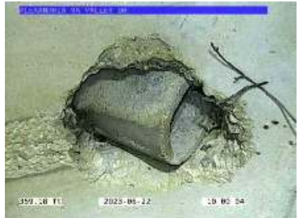
009388STMP_c7e1524c-cc60-44b4-9a64-ea9e11e6e0b4_20230622_103254_056.jpg, 00:07:52, 359.18ft Miscellaneous General Observation / PIPE CONNECTION
