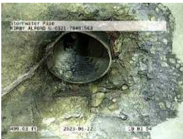
009388STMP_e114218d-37ca-43af-a568-5dc153d6c5ac_20230622_103354_520.jpg, 00:08:46, 409.03ft Miscellaneous General Observation / PIPE CONNECTION
