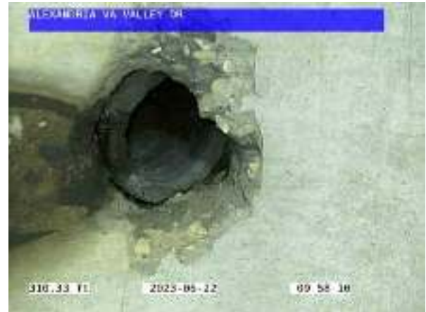
009388STMP_9edef05f-133f-49de-bf4a-1a0d692d42e2_20230622_103100_160.jpg, 00:06:27, 310.33ft Miscellaneous General Observation / PIPE CONNECTION
