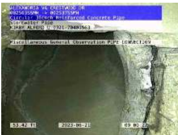
007462STMP_5cb1a6a0-3209-4565-89d0-37f327fbeadd_20230621_093309_534.jpg, 00:01:24, 53.42ft Miscellaneous General Observation / PIPE CONNECTION
