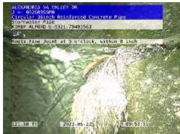
009388STMP_8cd6cad0-2ddc-4407-a58f-d2d4eb3e4051_20230622_102640_793.jpg, 00:02:44, 121.58ft Roots Fine Joint at 5 o'clock, within 8 inch
