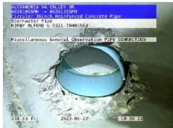
008792STMP_c398f669-1acf-4e39-aa92-5a73db30971f_20230622_111212_401.jpg, 00:05:14, 238.63ft Miscellaneous General Observation / PIPE CONNECTION
