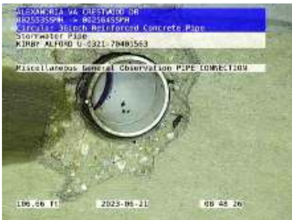
007464STMP_c753e772-de65-4a65-921c-7a0e3515459e_20230621_092113_847.jpg, 00:03:38, 106.66ft Miscellaneous General Observation / PIPE CONNECTION
