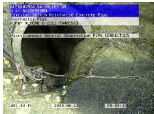
009388STMP_0990ec29-455a-487b-80a9-df60dab39b20_20230622_103202_841.jpg, 00:07:17, 341.43ft Miscellaneous General Observation / PIPE CONNECTION
