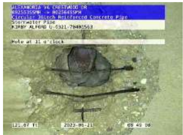
007464STMP_ee039985-5dcc-48ab-855a-c3b2a5833599_20230621_092155_768.jpg, 00:04:13, 121.68ft Hole at 11 o'clock
