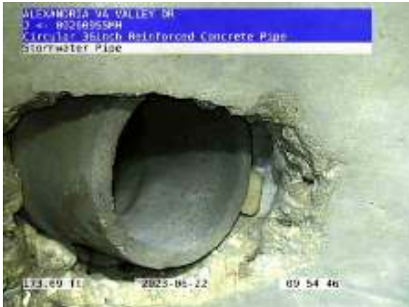
009388STMP_4efef903-8e99-4cda-a62b-1278e7569f0c_20230622_102735_752.jpg, 00:03:32, 173.69ft Miscellaneous General Observation / PIPE CONNECTION
