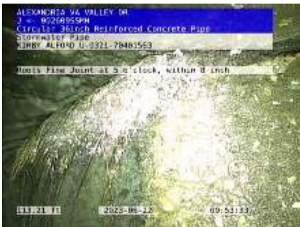
009388STMP_cd7635b1-5508-4e35-aadd-6589be399be7_20230622_102623_078.jpg, 00:02:30, 113.21ft Roots Fine Joint at 5 o'clock, within 8 inch
