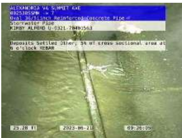
009064STMP_5e88708d-a199-4822-84c4-6fce5eae4744_20230621_095852_438.jpg, 00:00:56, 25.28ft Deposits Settled Other, 5% of cross sectional area at 6 o'clock / REBAR
