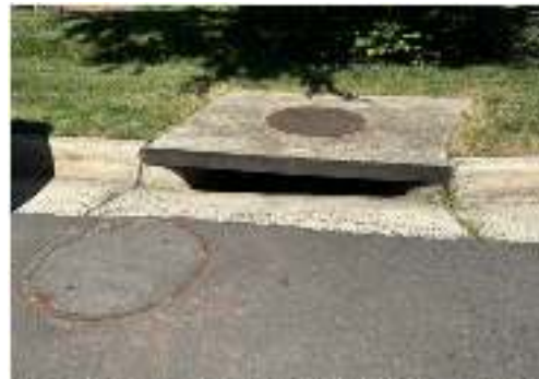
Photo 2: Storm drain pipe that flows south contrary to GIS direction
