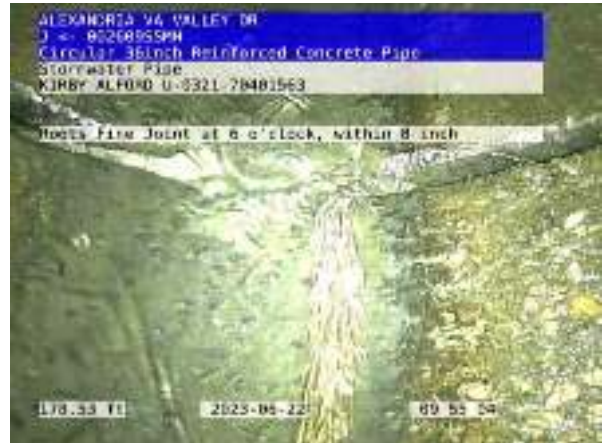
009388STMP_2c17cce2-d41c-471f-b23f-71b011b400c5_20230622_102753_488.jpg, 00:03:44, 178.53ft Roots Fine Joint at 6 o'clock, within 8 inch
