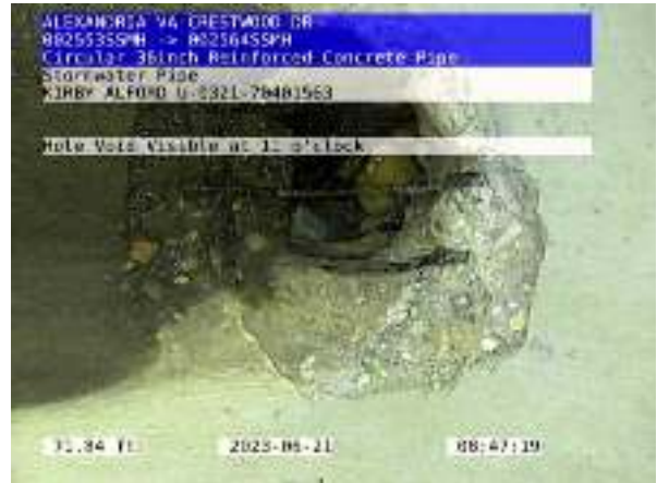
007464STMP_fefbbdb5-ffff-40e0-aba7-c4333ea9ea5a_20230621_092006_345.jpg, 00:02:39, 71.84ft Hole Void Visible at 11 o'clock
