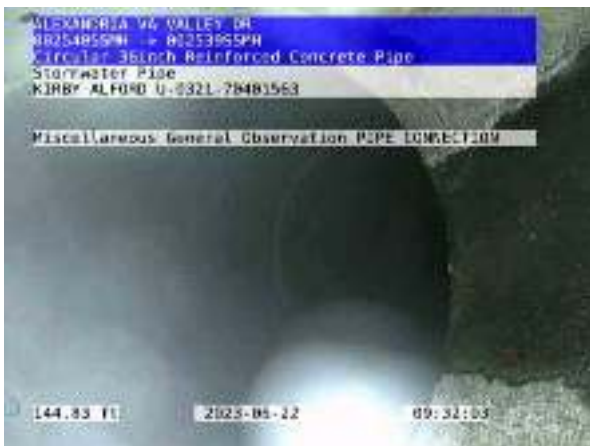
009067STMP_e39816e4-7749-4060-bac7-6f39f8314072_20230622_100452_667.jpg, 00:02:58, 144.83ft Miscellaneous General Observation / PIPE CONNECTION
