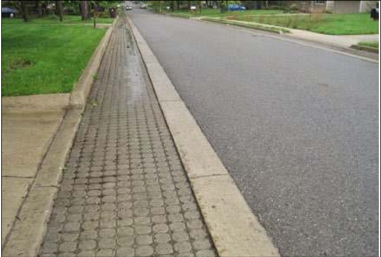
Figure 11.10. Green infrastructure practice: permeable pavers (USEPA 2021).
