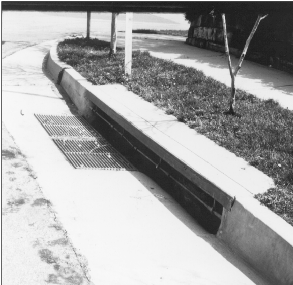
Figure 7.12. Sweeper combination inlet.
