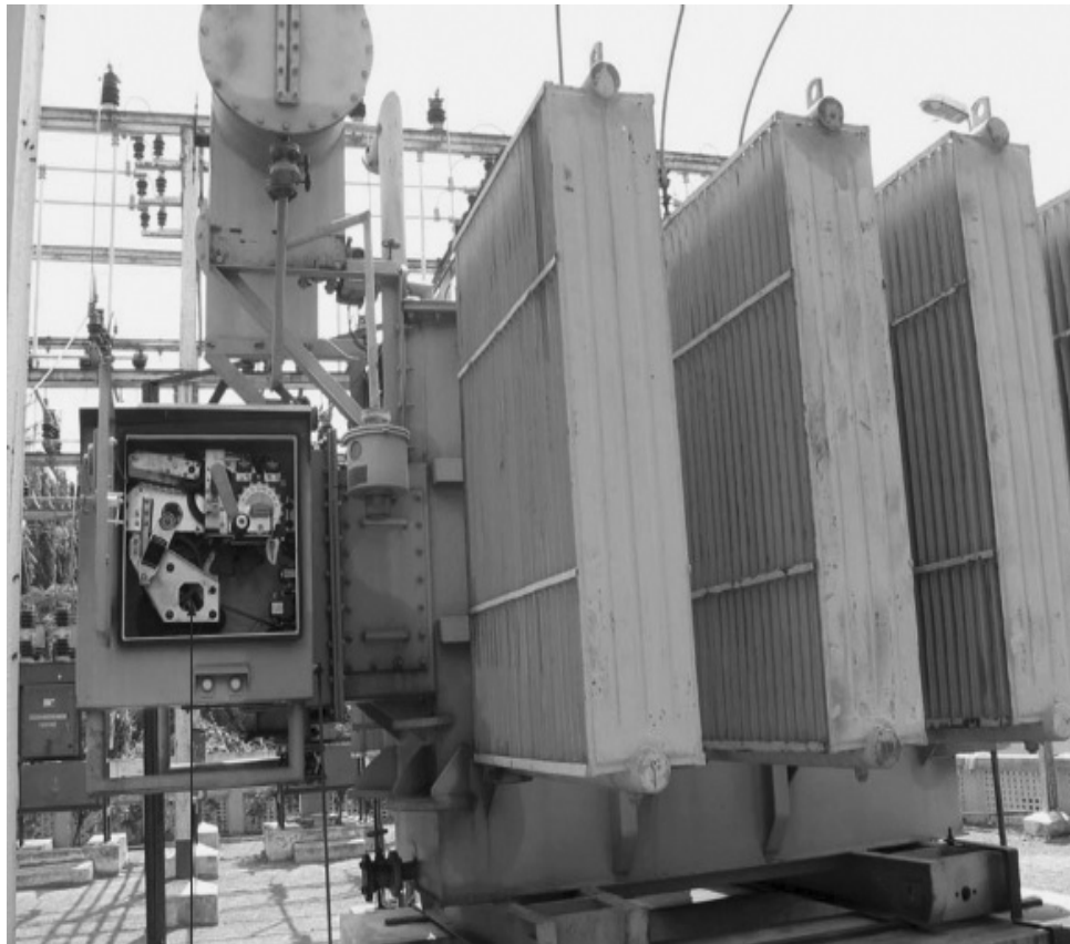
View of on-load tap changing of 2.5-MVA transformer
