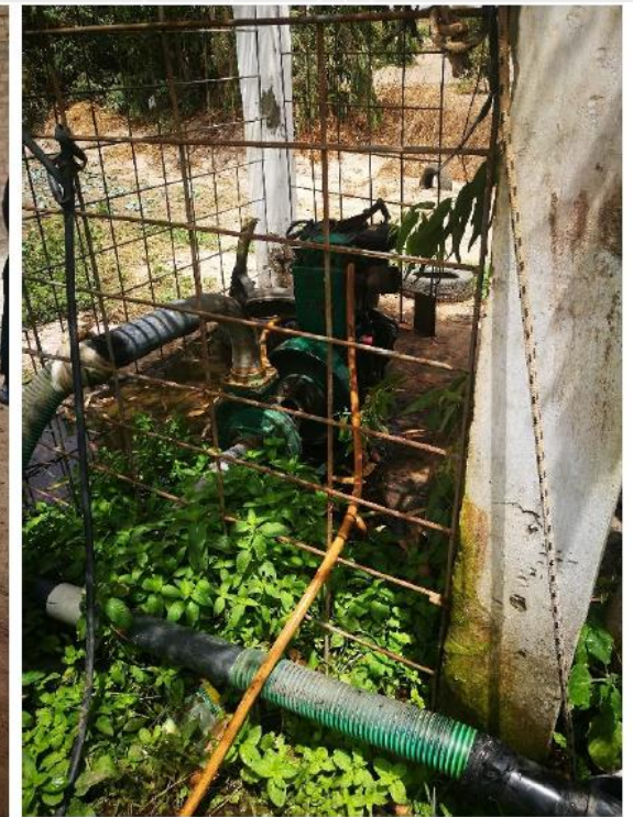
Borehole (with electric pump)
