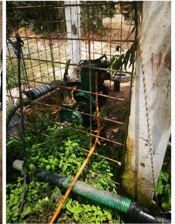
Borehole (with electric pump)
