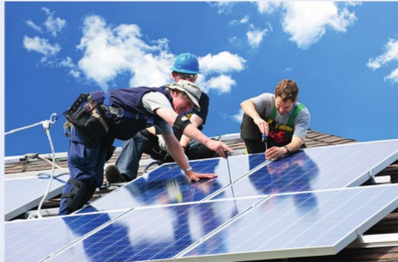
▲ Solar power installation
